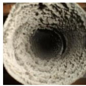
Fig. 2 Dust adhered in the duct
